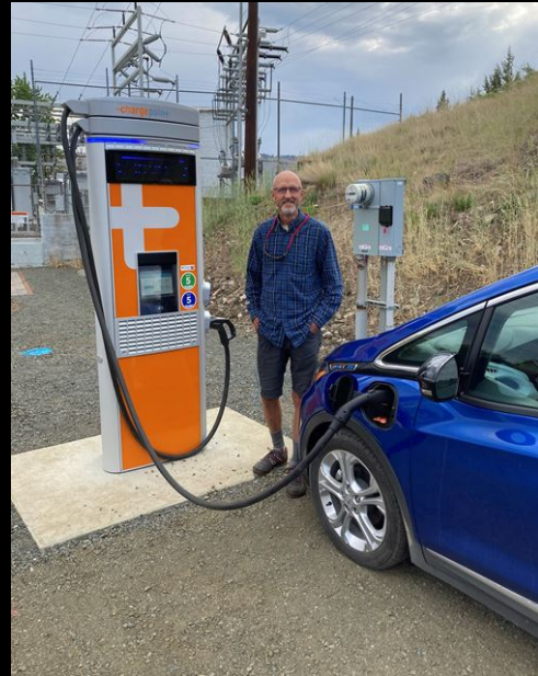
Second EV Charging Station Installed In John Day
